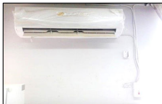
Figure 3: Air conditioning unit is separate and not central.
