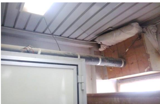
Figure 2: Incorrect installation of gas and vapours tubes which may lead to leakage.
