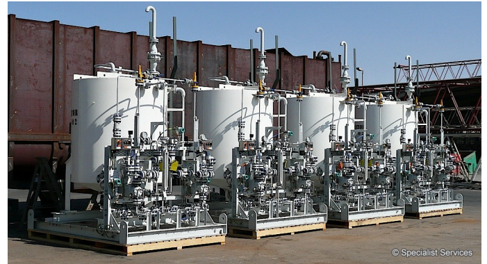
Figure 5. Chemical Injection Machinery.
